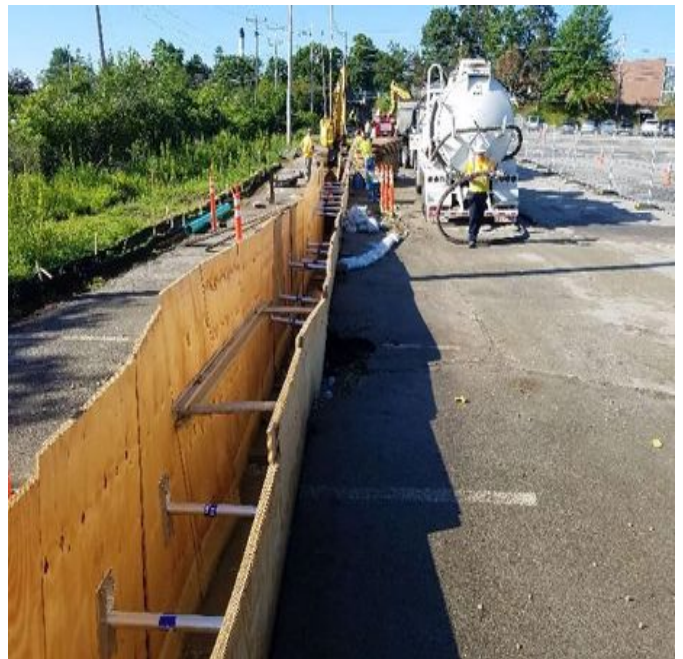
Fig 4: Pump truck used to pump out rain water from trench in "A" lot. Viewing south. (6-17-19).
