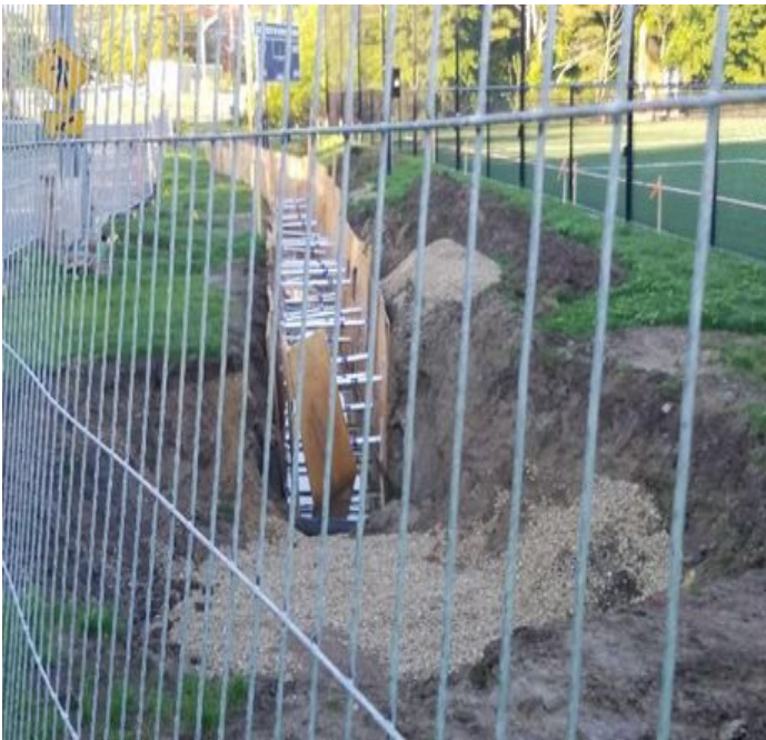
Fig 3: Rain water present in trench along Colovos Rd, UNH. Viewing south. (6-17-19).
