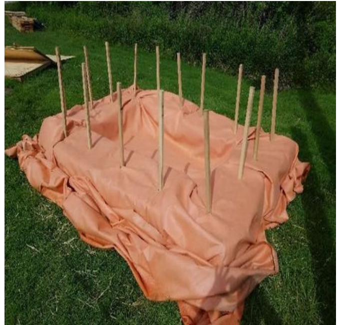
Fig 2: Dewatering apparatus installed along Colovos Rd, north of College Brook, UNH. Viewing northeast. (6-14-19).
