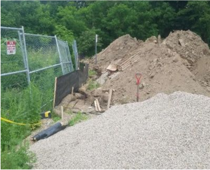
Fig 9: McCourt installed silt fencing and straw waddle between the soil stockpile In Waterworks Rd and wetland DW65. Maintenance needed, see above. Viewing east. (6-17-19).
