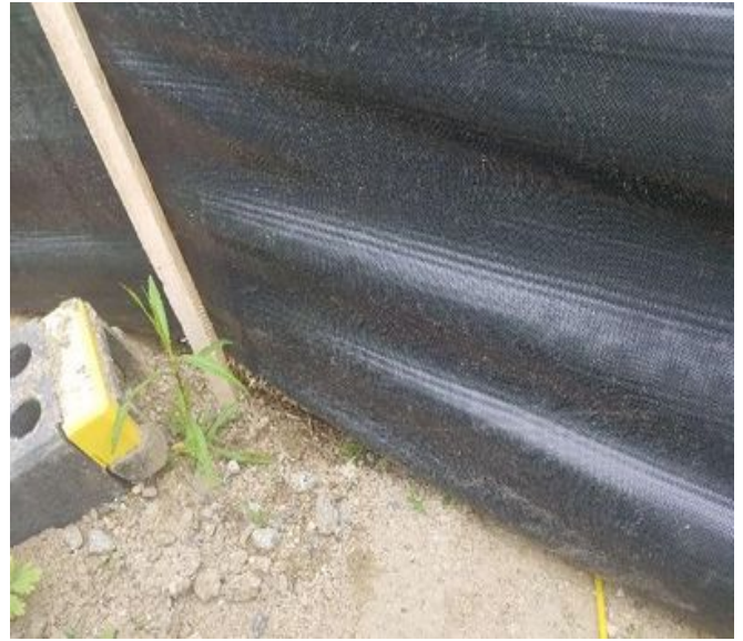
Fig 10: Silt fence installed in the Waterworks Rd laydown area needs to be keyed into the ground, see above. Viewing east. (6-18-19).
