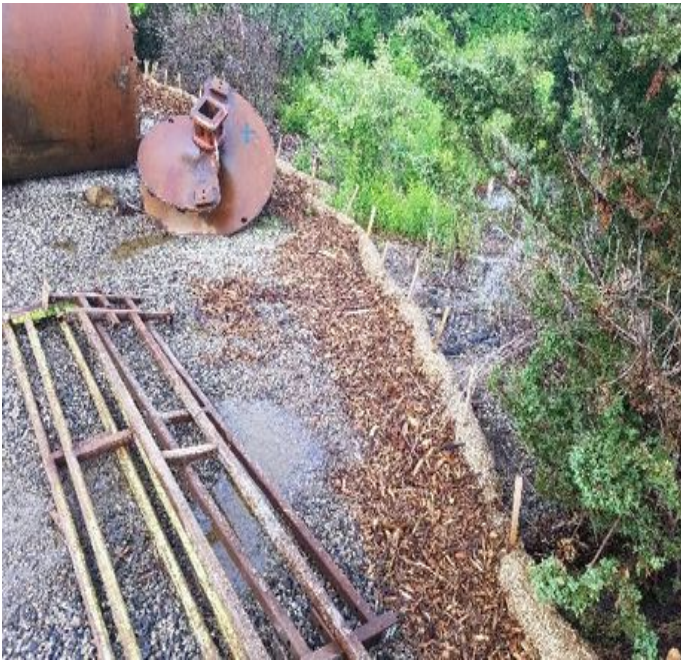
Fig 1: Combined berm installed around laydown area off of Gosling Rd. Viewing south. (6-14-19).
